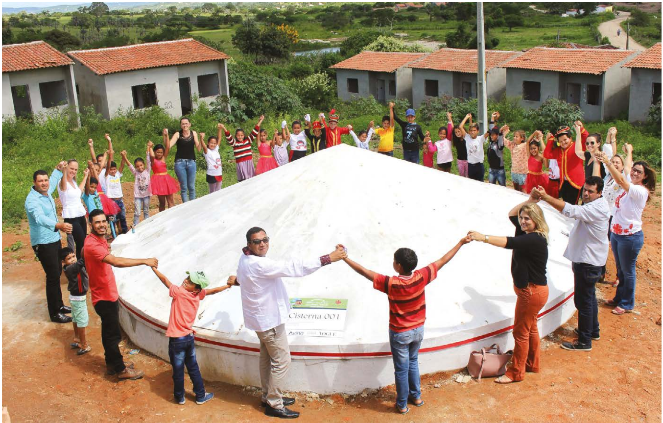
Construction of a 52,000 litre plate cistern, water-reuse system, with vegetable garden and orchard in Massaranduba, Poçoão in the Brazilian semi-arid region
